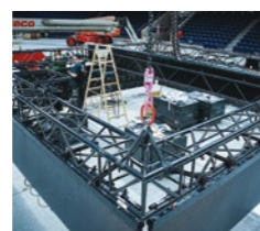
LED-Cube in Braunschweig (Foto: Ledcon)
